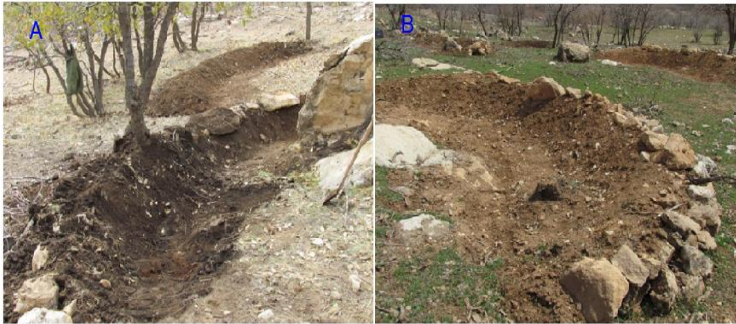
Fig. 2. The constructed crescent shaped infiltration trench in the study area at the first year (a) and using fragmented rock in embankment wall (b)
