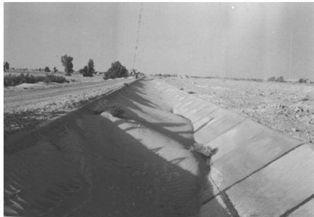
Fig. 7. Accumulation of sand in the irrigation canal
